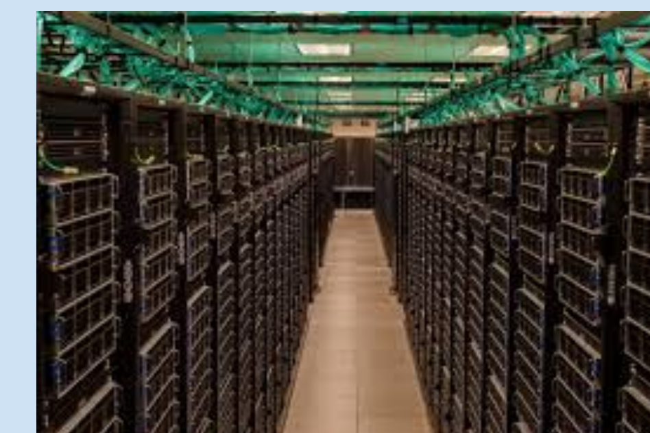
The Frontera Supercomputer at TACC -- #8 in Top 500
